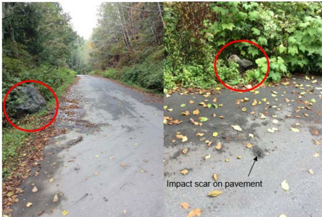
Figure 4-4. Fresh (charred) boulders observed in downslope ditch of Zeballos Main Road. Photographs by BGC, September 13, 2018.
