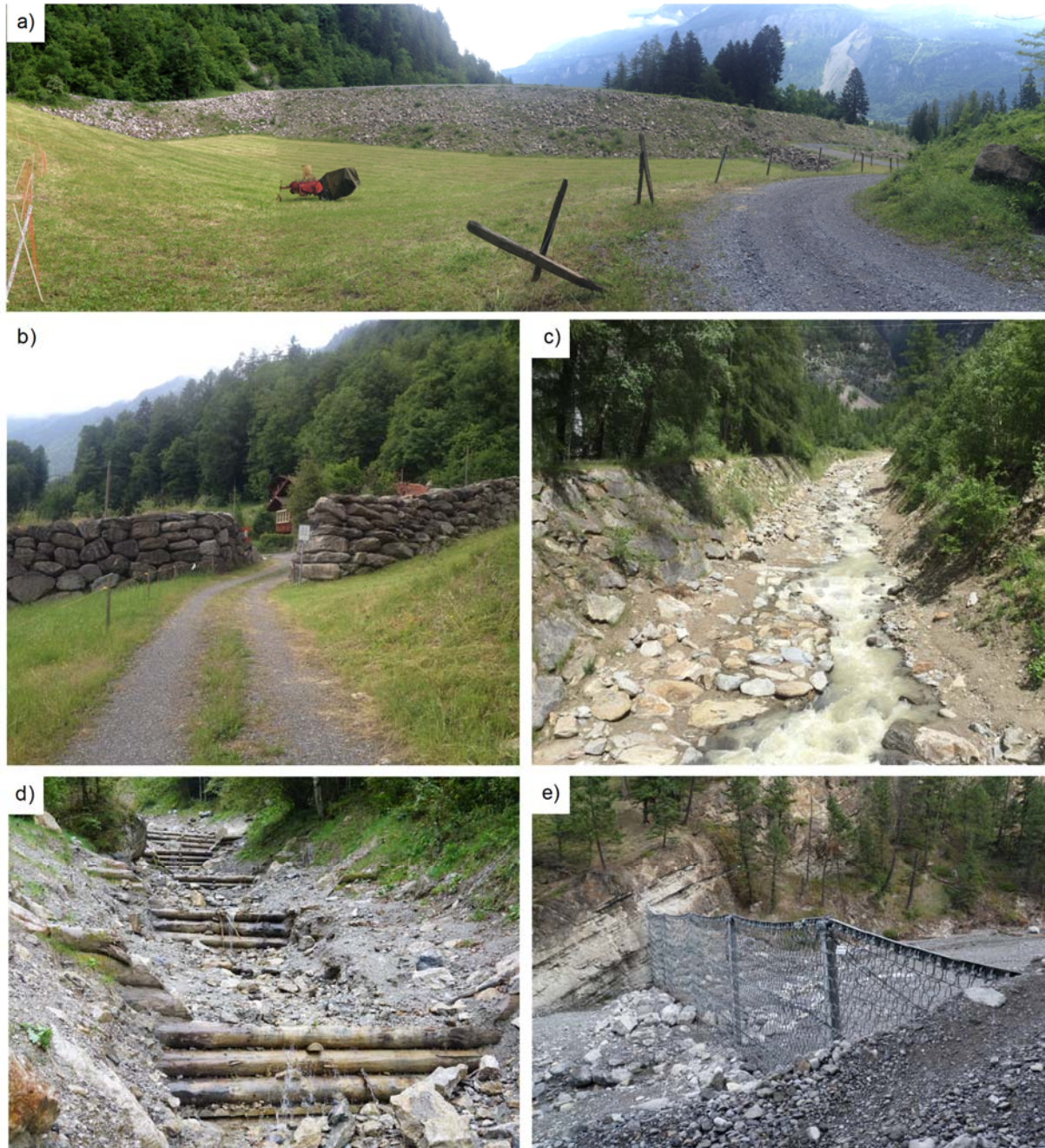
Figure C-1. Examples of debris-flow mitigation structures: (a) an earth-fill retention berm on Glyssibach, Brienz, Switzerland; (b) a stone diversion berm, Trachtbach, Brienz, Switzerland; (c) a conveyance channel with earthfill berms, Rennebach, Austria; (d) log crib check dams, Gesäuse, Austria; and (e) a flexible debris net for debris flood mitigation, Cougar Creek, Canmore, Alberta. Photograph (d) by M. Jakob, other photographs by E. Moase.
