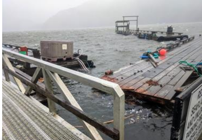
Figure 11 - Storm damage at the municipal airplane dock, and fuel dock
