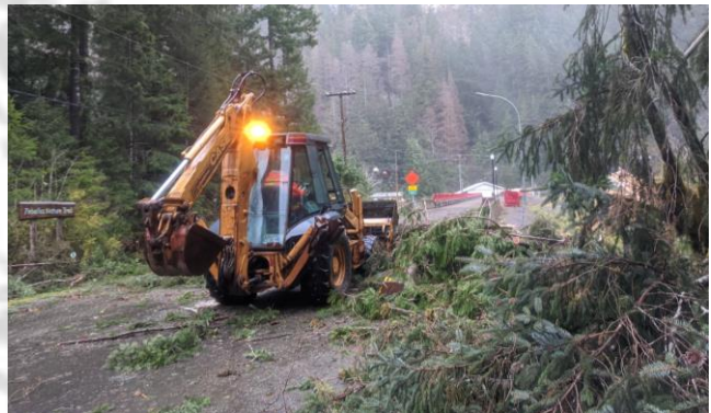
Figure 12 - Public Works Staff clear tree debris near the Sugarloaf Bridge
